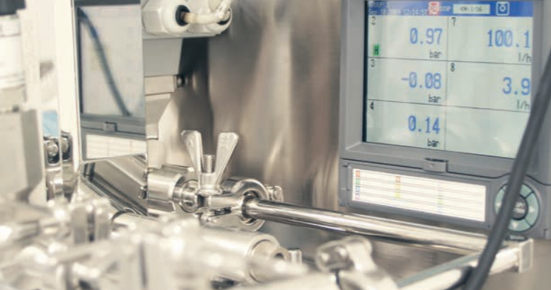
Close-up of large scale UF/DF control unit
